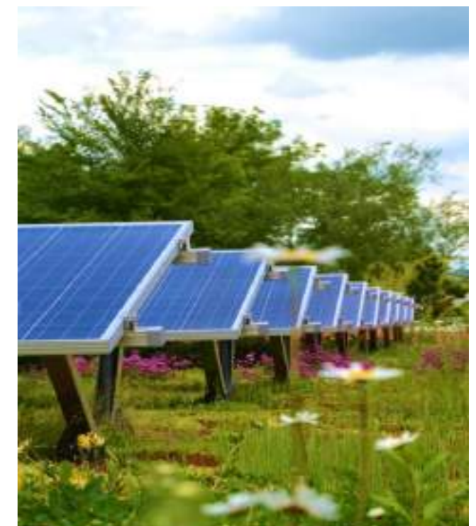
Figure 9.16 Green flat roof with PV panels © Contec
