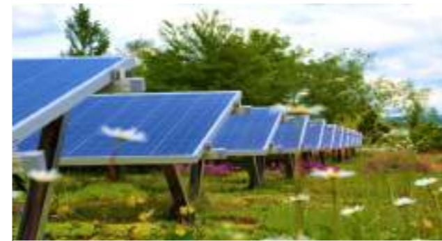
Figure 2.6 Green Flat Roofs with PV systems © Contec
